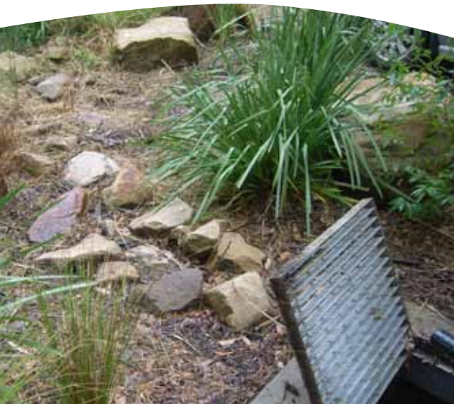
Rock lined channel through the garden bed, and into one of the three inlet pits (bottom right)
