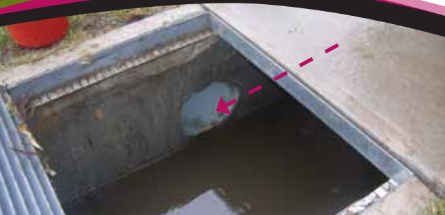
Stormwater overflow pipe which discharges directly in the Parramatta River
