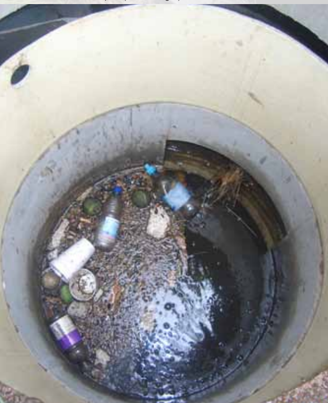
Litter and debris captured inside the treatment unit
