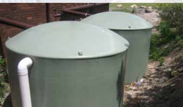
10kL rainwater storage tanks located at the back of the Sailing Club (connector pipes from the roof shown in the background)
