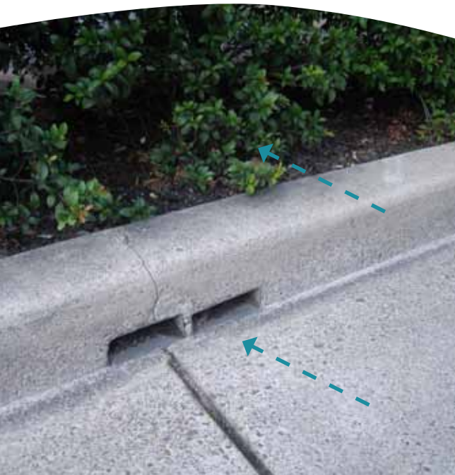
Inlet slots along Church Street gutter. Hedge vegetation of the garden bed in background.
